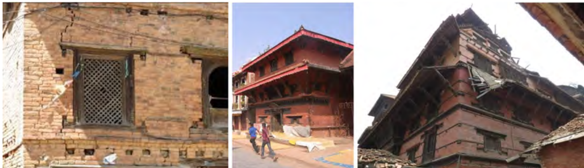
Figure 5: (left) The framed window [9 – Kathmandu 2015]; (center) timber corner stitch element (S. Tonna, 2011 – Baktapur); (right) the timber bands at each floor [9– Kathmandu 2015].
