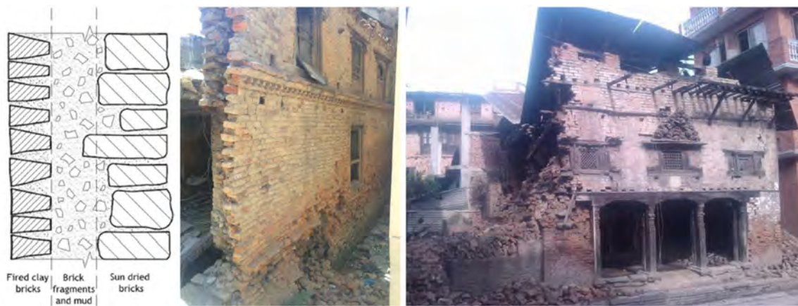
Figure 2: Masonry details: (left) a sketch of a hypothetical arrangement of layers in the wall thickness (Authors for the purpose of the article, 2019); (central) 2015 Earthquake effects on masonry walls [9 – Bagmati 2015]; (right) 2015 Earthquake effects Baktapur [10 – Baktapur 2015].
